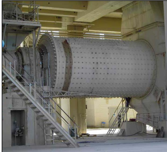
Figure 3.2.76 Cement grinding. Holcim Cement Plant, Spain.
