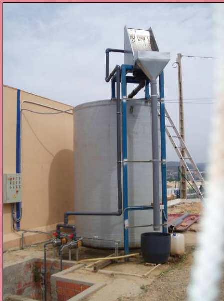
Final discharge treatment installation: Double pump (1+1), final sieving and aerated homogenisation
